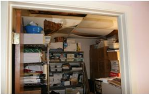
Office Area and Storeroom after Ike
